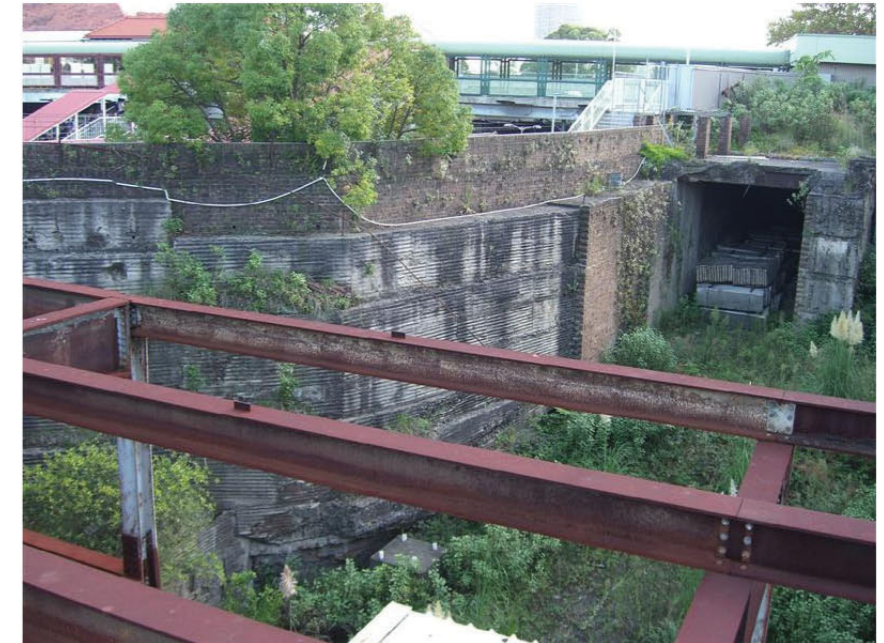
21. From the car park looking towards Sydney across the void. the concourse is visible over the brick and concrete retaining wall. The "country" portal of the Down Southern Suburbs Dive is also visible.
