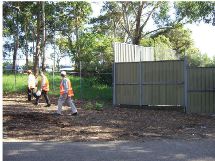
28. Looking towards Sydney from the park. The sheet piling at the end of the Up Southern Suburbs Tunnel is ~ 6m beyond the chain wire fence.
