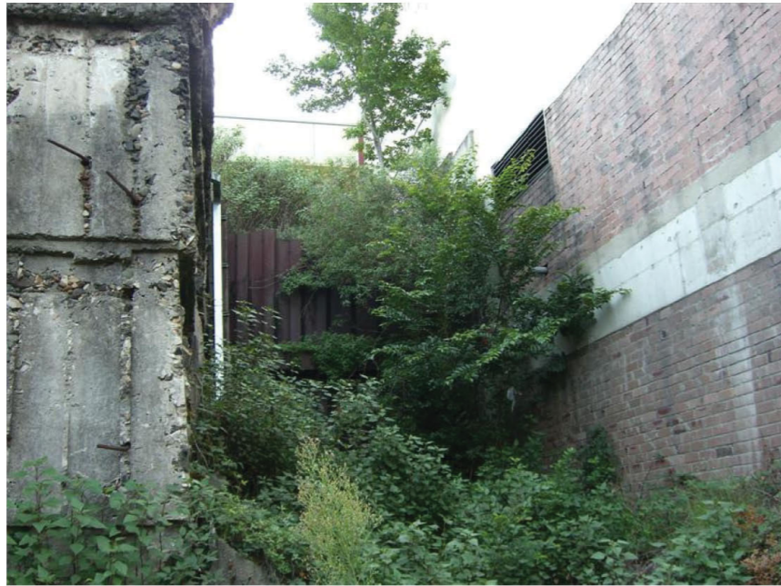
7. Space between the country portal of the Down Southern Suburbs Dive (left) and the entrance building for platforms 11 & 12 (right)
