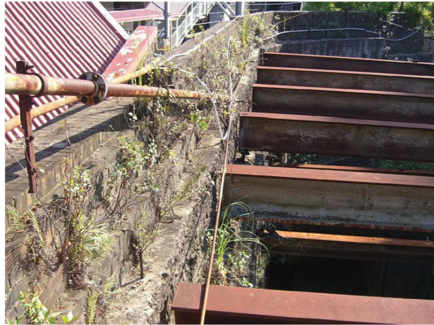
19. From the car park looking towards Sydney at the top of the brick and concrete wall between platform 10 and the void. The roof of the heritage building on platform is visible to the left.
