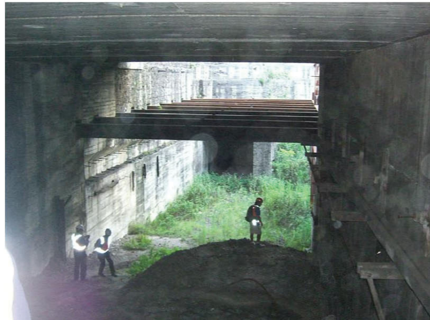
16. Looking from the Southern Suburbs "tunnel" towards Sydney. the country portal of the Up Southern Suburbs Dive is visible immediately below the steel beams.
