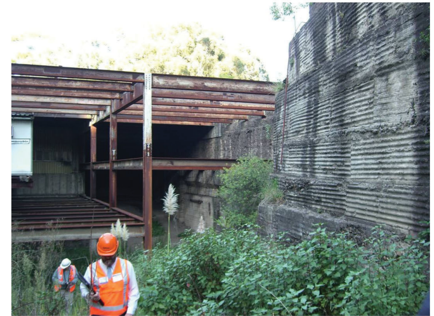
5. Within the void looking away from Sydney from the "country" portal of the Down Southern Suburbs Dive.
