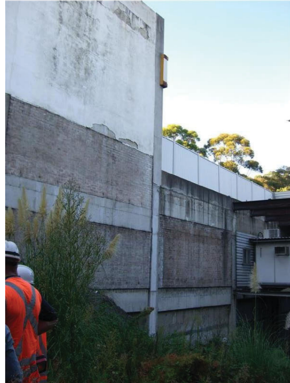
3. Within the void looking at the western wall of the mezzanine level above platforms 11 & 12
