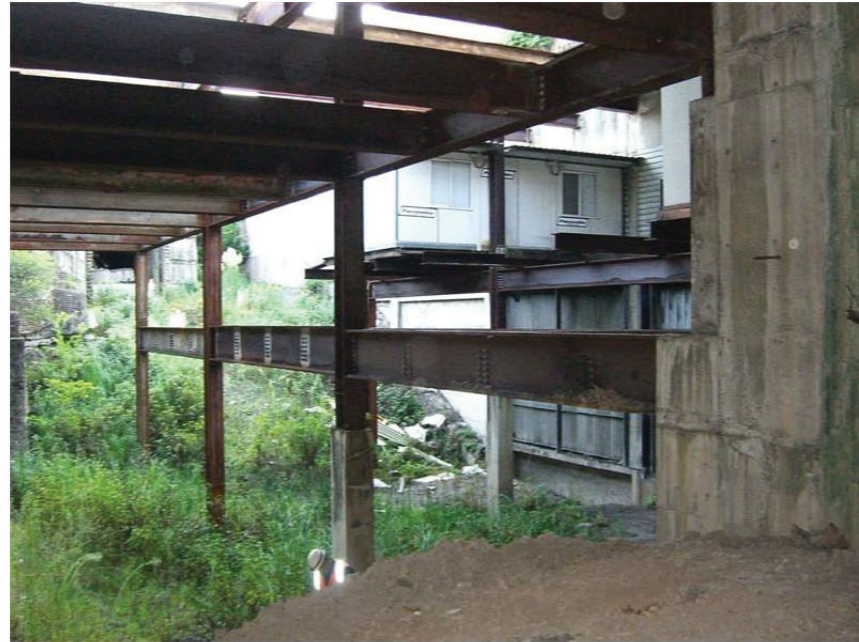
15. Steel beams within the void looking from the Southern Suburbs "tunnel" towards Sydney.
