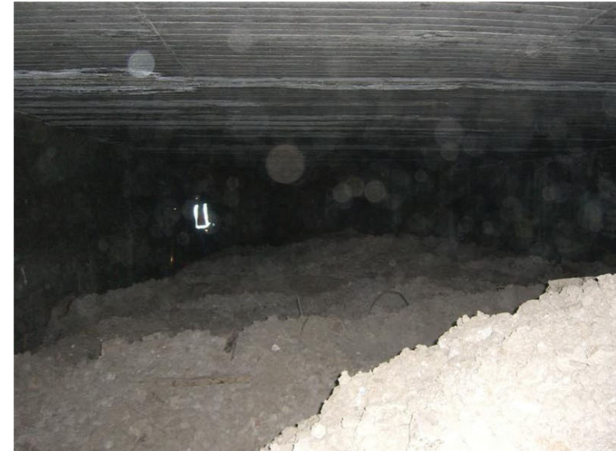
17. Up Southern Suburbs "tunnel" looking away from Sydney. The spoil is stacked quite high in the far section of the tunnel.
