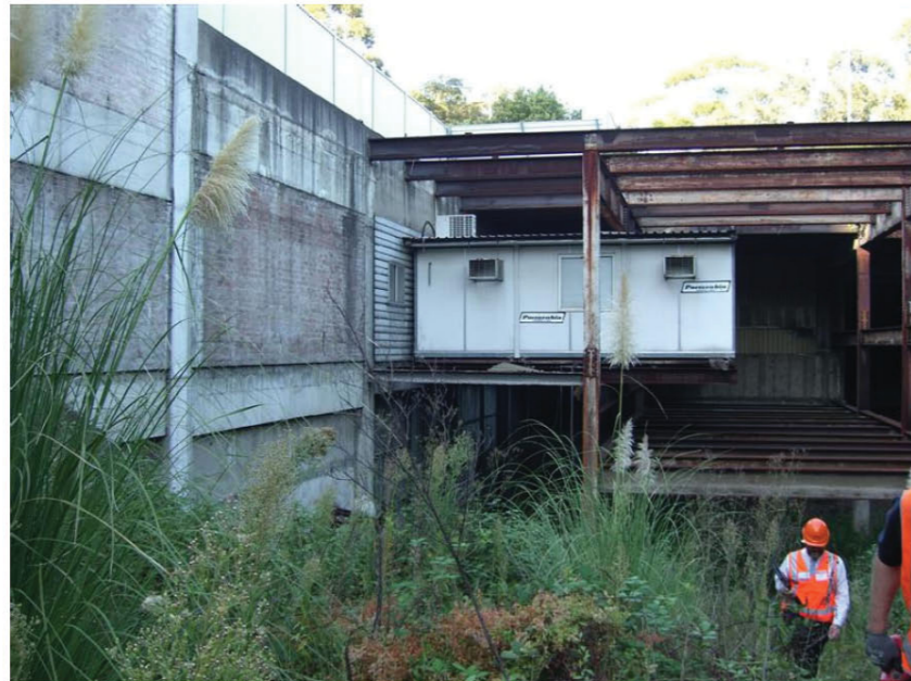
4. Within the void looking away from Sydney from the "country" portal of the Down Southern Suburbs Dive.
