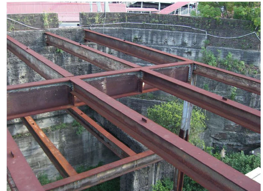
22. From the car park looking over the steel beams above the void. The "country" Portal of Up Southern Suburbs Dive is visible below the beams.
