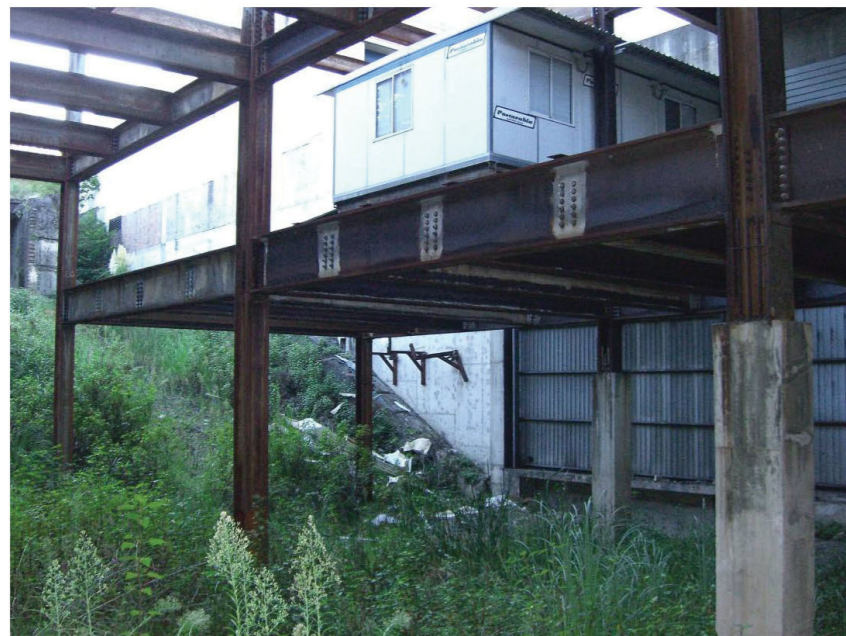
12. Portable building positioned on steel beams in the void at mezzanine level.
